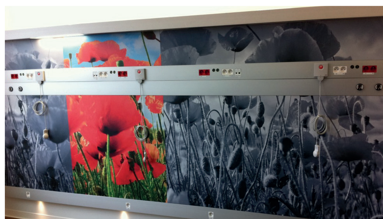
Centre Hospitalier, Ath - Belgique Hospital Center, Ath - Belgium
